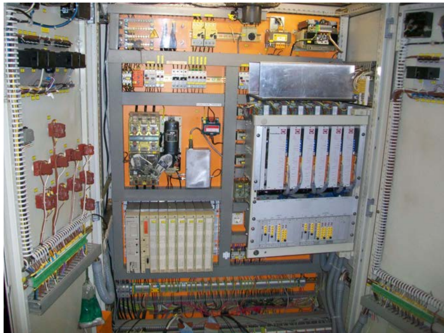
Figure 17: The Azimuth drive electronics exhibited a fault that was beyond our immediate ability to repair.
