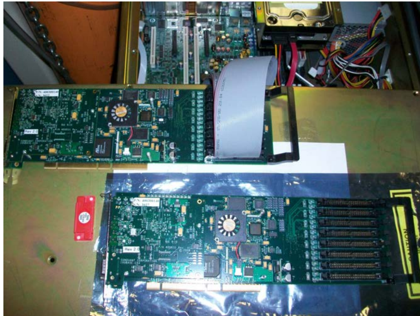
Figure 16: The faulty amazon card (still cabled) and the replacement (uncabled) are shown. The IDE cables were swapped from the old to the new card and operability was restored.
