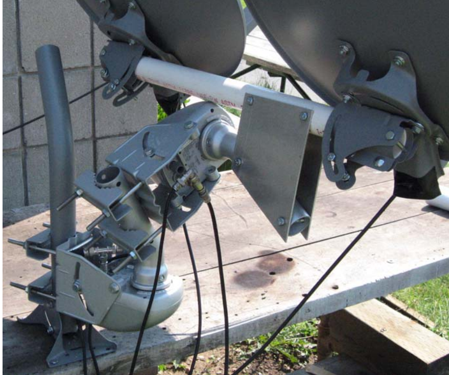
Figure 3.2.2: VSRT rotation system controlling two adjacent dishes
