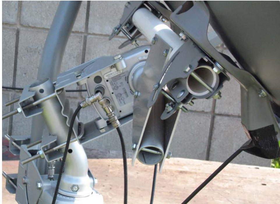
Figure 3.1.3.1: Coaxial cables installed on dish structure
