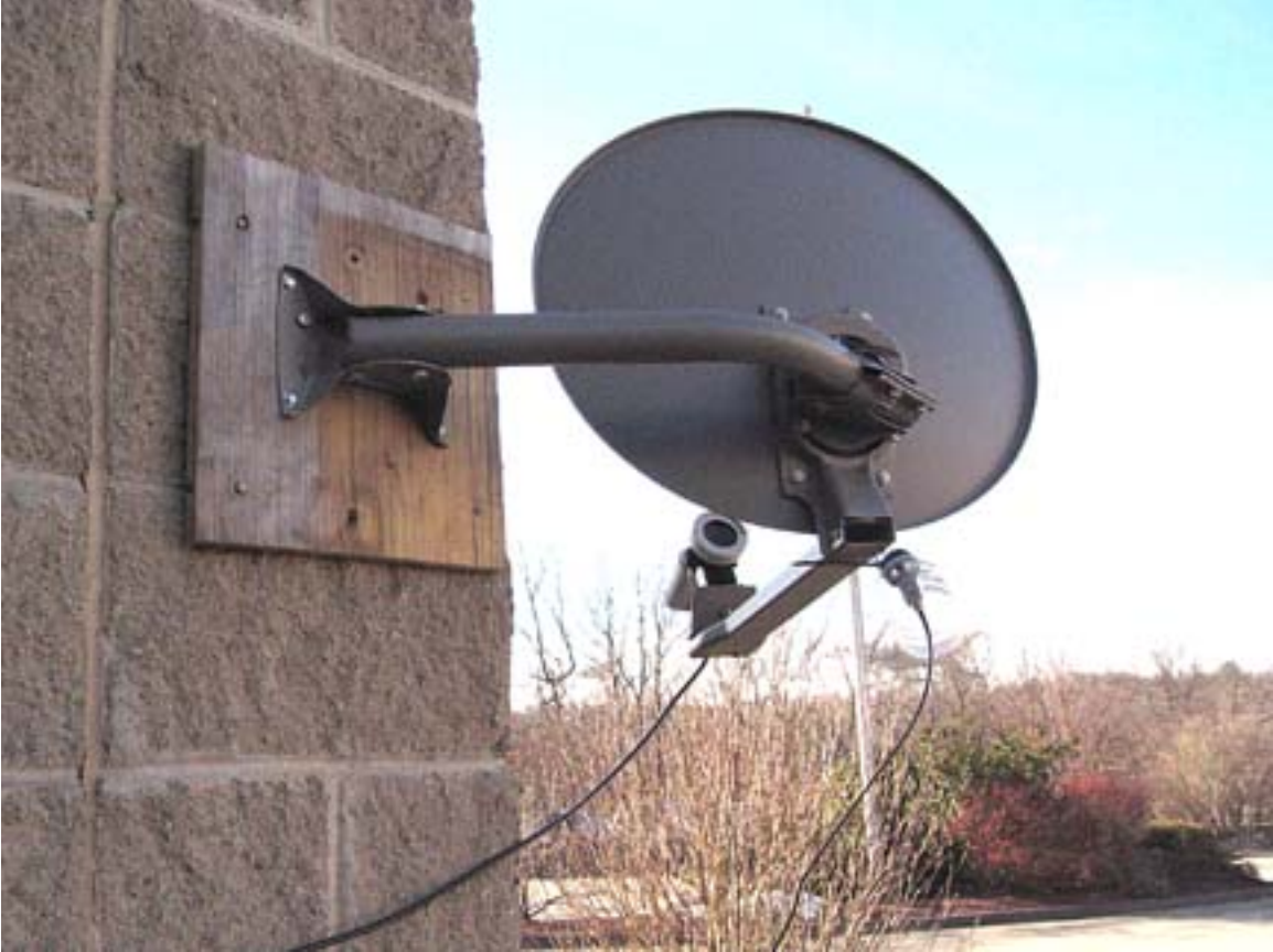
Figure 3. Rear view of the dish showing the frequency calibration probe and the mounting to the building wall. The cables from the LNB and the calibrator are about 10 feet long. [It is highly desirable to keep the cable to the LNB as short as possible.]
